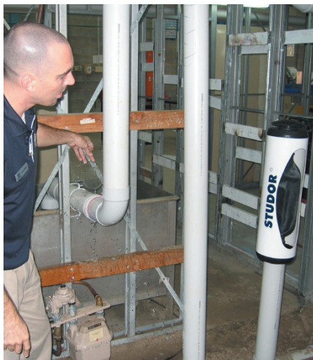
David Griffiths of Studor Australia demonstrates the power of P.A.P.A. to building designers, engineers and consultants at the Gore Hill TAFE rig earlier this year.
